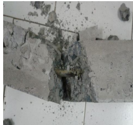
Figure 17 Failure of singly reinforced slab panel
